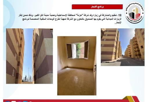
Organizing a visit site for a delegation from Khazna Company to Ismailia Governorate in preparation for offering the housing units allocated for the rental program
